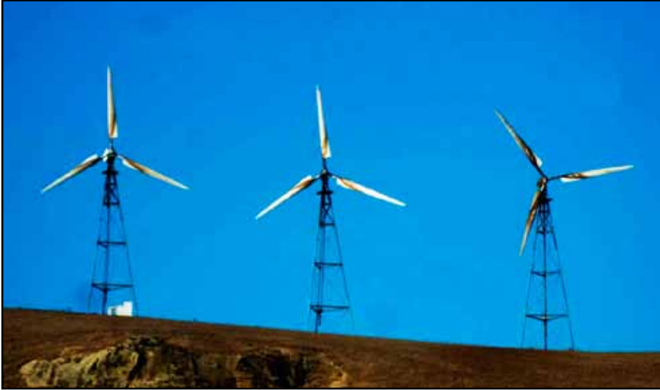
Decrepit turbines owned by Altamont Winds, Inc., showing streaks of oil, leaking from the generators, on the vanes. Photo: Final Supplemental Environmental Impact Report 2018 CUP Extension.
